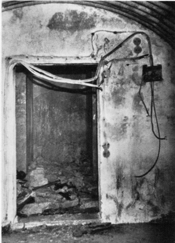
As recorded in 1975 the inside of Ardingly Zero Station showing wiring still in place and entrance shaft in background. Photo Harry Townsend
